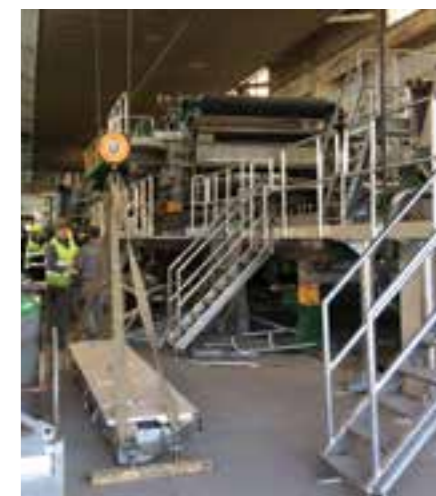
Prenovljeni mokri del KS2 med prenovo Renovated wet end of the KS2 cardboard machine during renovation
